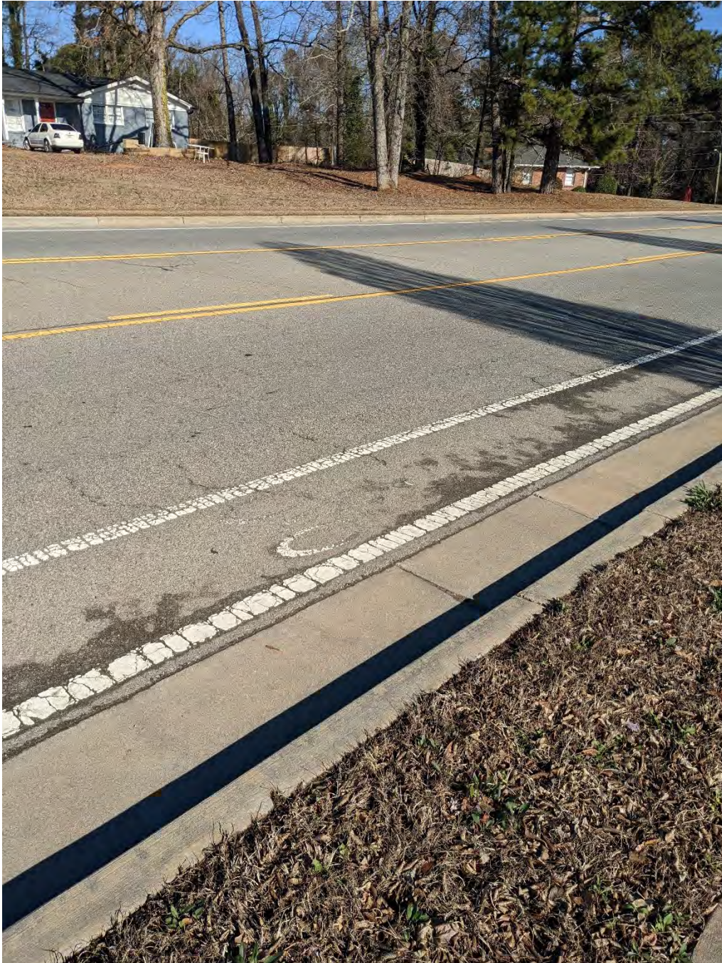
FIGURE 19: BIKE LANE ALONG KENNESAW DUE WEST RD, BETWEEN BURNT WOOD DR AND COBB PKWY
